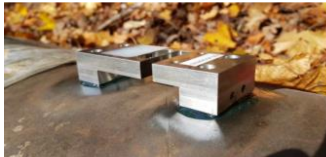
Fig. 8: SENSOCOF sensible element installed on the penstock.
