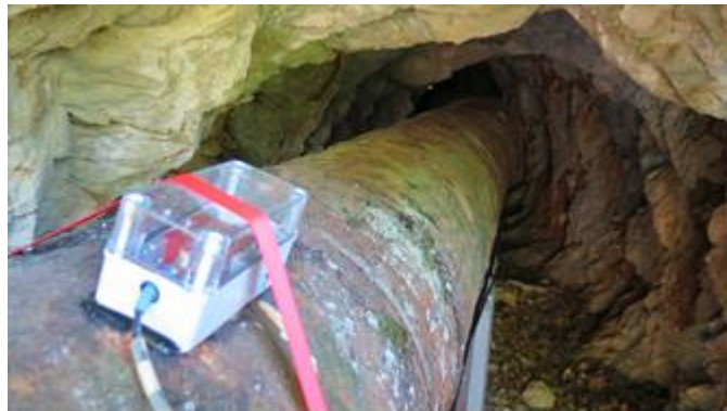
Fig. 3: An AE sensor and its preamplifier installed inside a protection box in a tunnel section.
