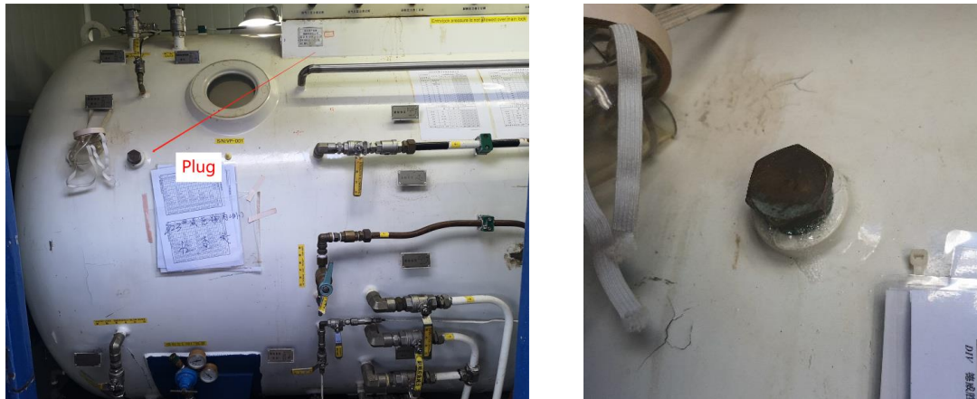
Fig. 10: Plug and when it leaked slightly.
